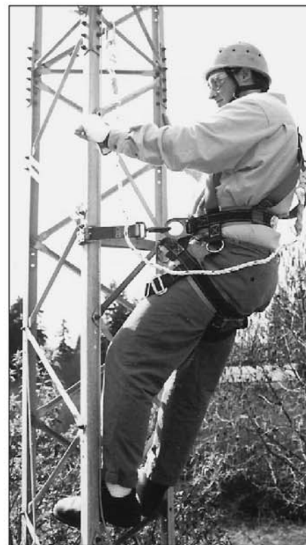
Figure 3 — The fall arrest lanyard is above the climber so that the climber can climb up to it. The fall-arrest and positioning lanyards are then "leapfrogged" so that the climber remains attached to the tower 100 percent of the time.
