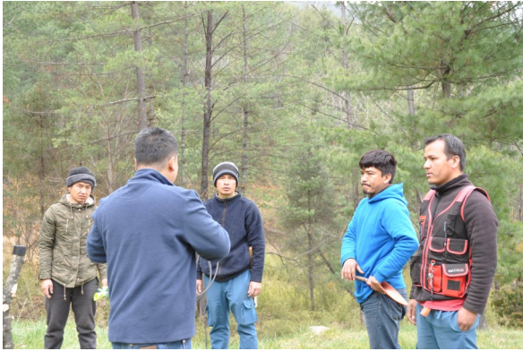
Young Bhutanese men are helping with antenna installation under Champ's (E21E1C) supervision
