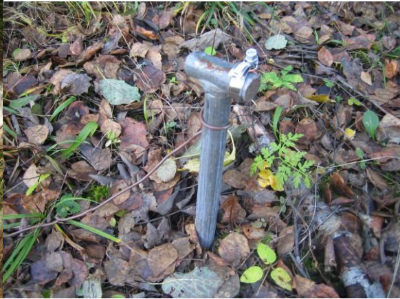
Grounding rod in NW end.
