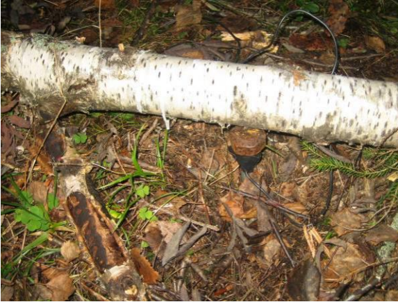
Camouflaged grounding rod at East end
